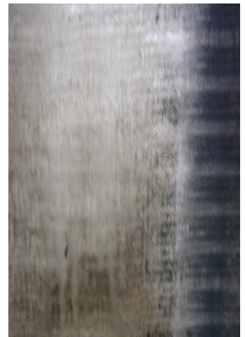
Condenser coil fouled with dust, dirt and vehicle exhaust particles. This caused increased electrical consumption in the air-conditioning system.
