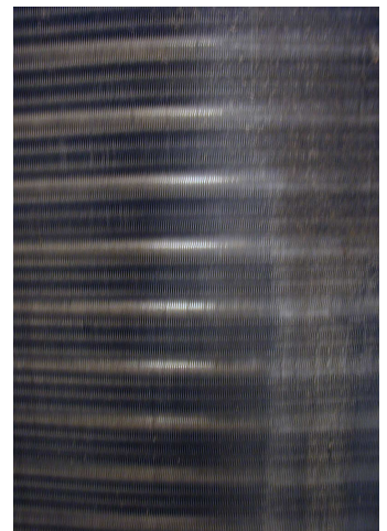
Same coil after one cleaning with NuCoil 145, a neutral coil cleaner produced by International Chemtex Corporation. System is now operating efficiently and has no difficulty in meeting cooling demand. Savings were estimated at 15 to 20%;
