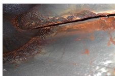
SRB pitting in a carbon steel filter housing
