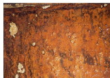
SRB nodules and pits on chiller end bell
