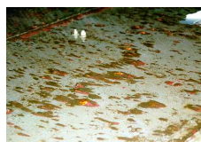
Active SRB nodules in cooling tower basin
