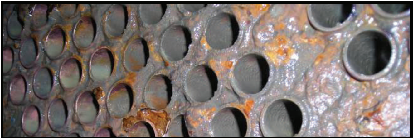
A scaled chiller from a system treated with a mechanical device.
