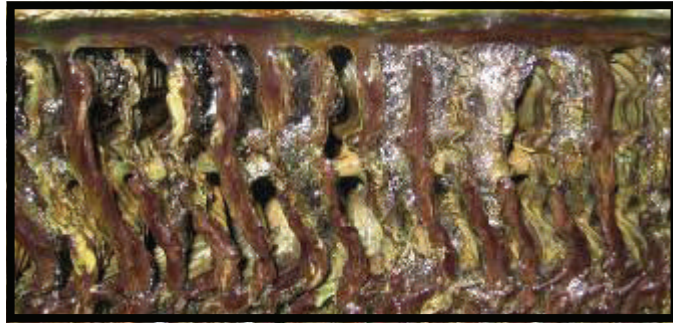
Microbial growth in the tower fill of a mechanically treated system.
